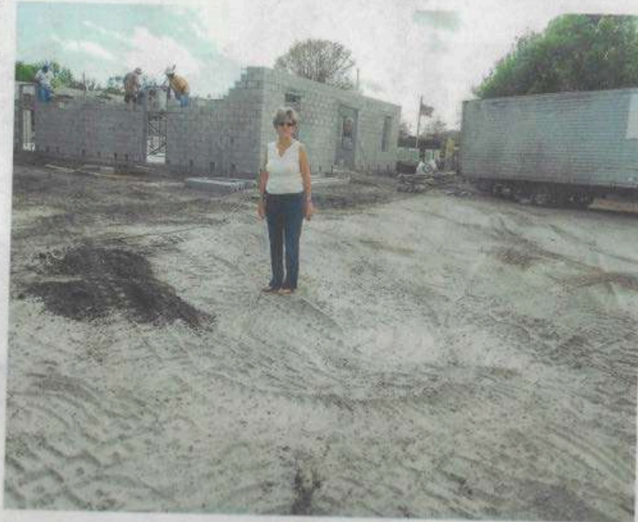
Shelly Ferger, foreground, stands in front of the administrative and training center being built at the Dog Park in Vero Beach by Dogs For Life.
